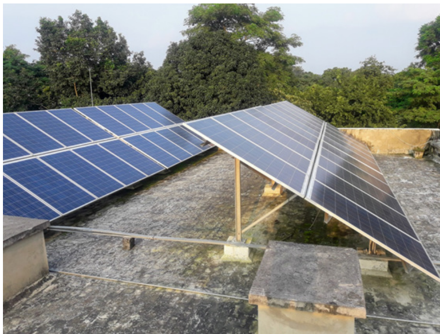
Fig.1 Solar Photovoltaic (SPV) panels installed at the rooftops
